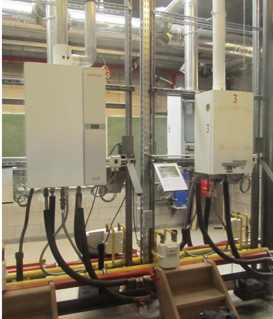
Control units, EFB VET College workshop, Brussels
